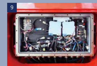
Electrical control system
